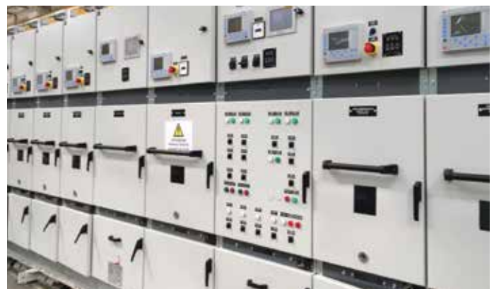
MV Main Switchboard with Shock Withstand Requirements 12kV - 630A - 31,5kA LHD - Italian Navy
