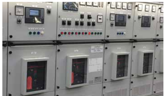
LV Main Switchboards with Shock Withstand Requirement 690V - 4000A - 65kA PPA - Italian Navy
