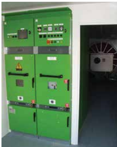
LV Shore Connection Panel 690V - 2500A - 100kA LSS - Italian Navy
