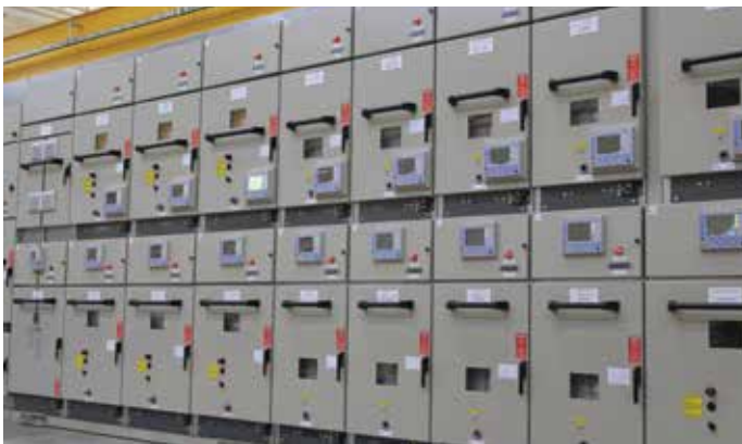
MV Main Switchboard 11KV - 4000A - 50kA Internal Arc Proof with Is Limiter
